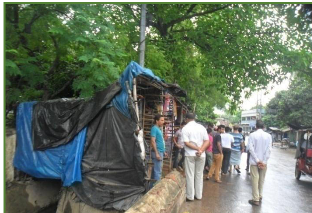
D4- Present condition of drain, Magura
