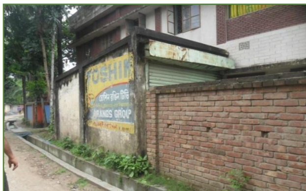
D8-Drain shifted to avoid the distortion of garage, Magura
